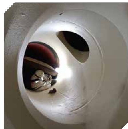
Main condenser scoop pipe for sea water intake
